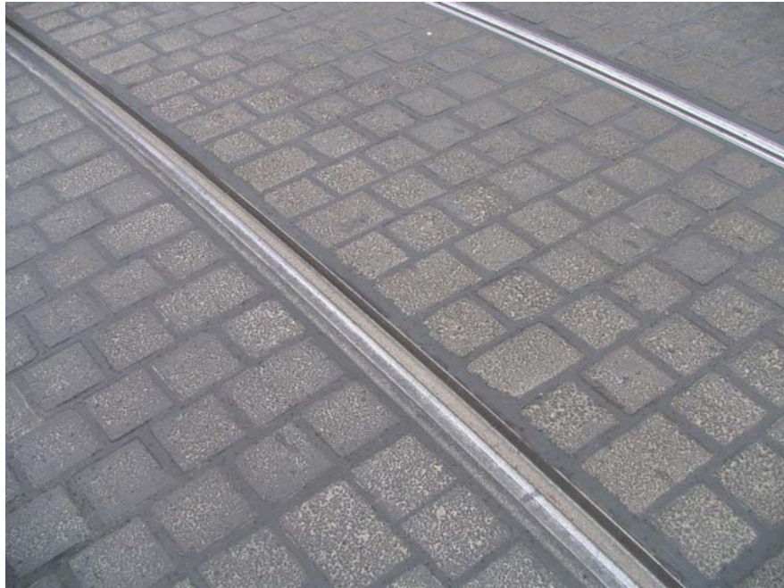
An example of street surface reinstatement using concrete blocks, with hot poured sealant between blocks and rail
