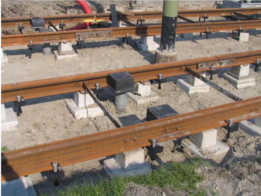
An example of traditional drain boxes for grooved rail prior to concreting in. J Snowdon
