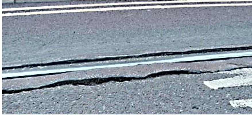
Lateral roll of rails causes road surface damage
