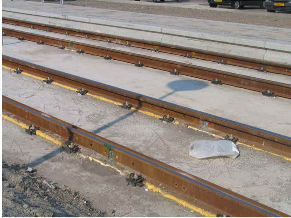
New track in The Hague, showing (nearest) expanding foam injected into the gap between the rail and the concrete.
