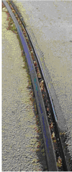
Welded repair to keeper flange - Fleetwood
